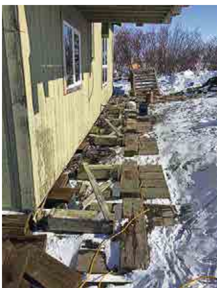
An earthquake shook this Selawik house off its foundation after years of erosion made it unstable.
